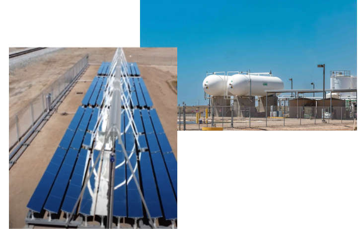
SunVapor's Two SHIP facilities for Dimethyl Ether Production & Almond Processing
