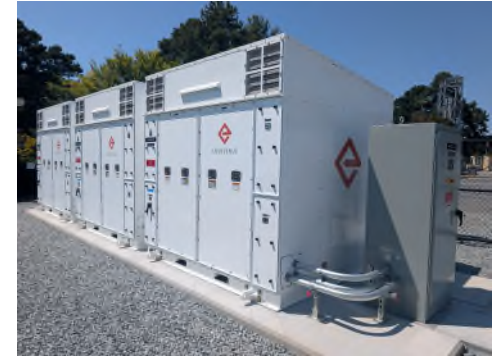
EnerVenue at Mt Holly Microgrid
