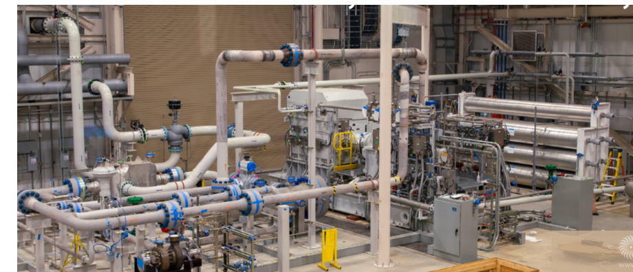
10 MWe STEP sCO 2 Pilot Plant
